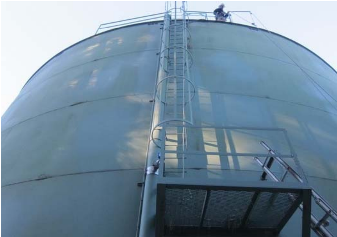
MG#1. Existing exterior ladder. There is no existing fixed portion of ladder below the platform.
