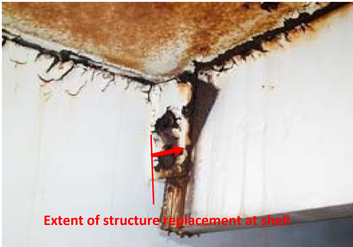
MG#2 existing rafter and shell clip and extent of roof structure replacement at the shell.
