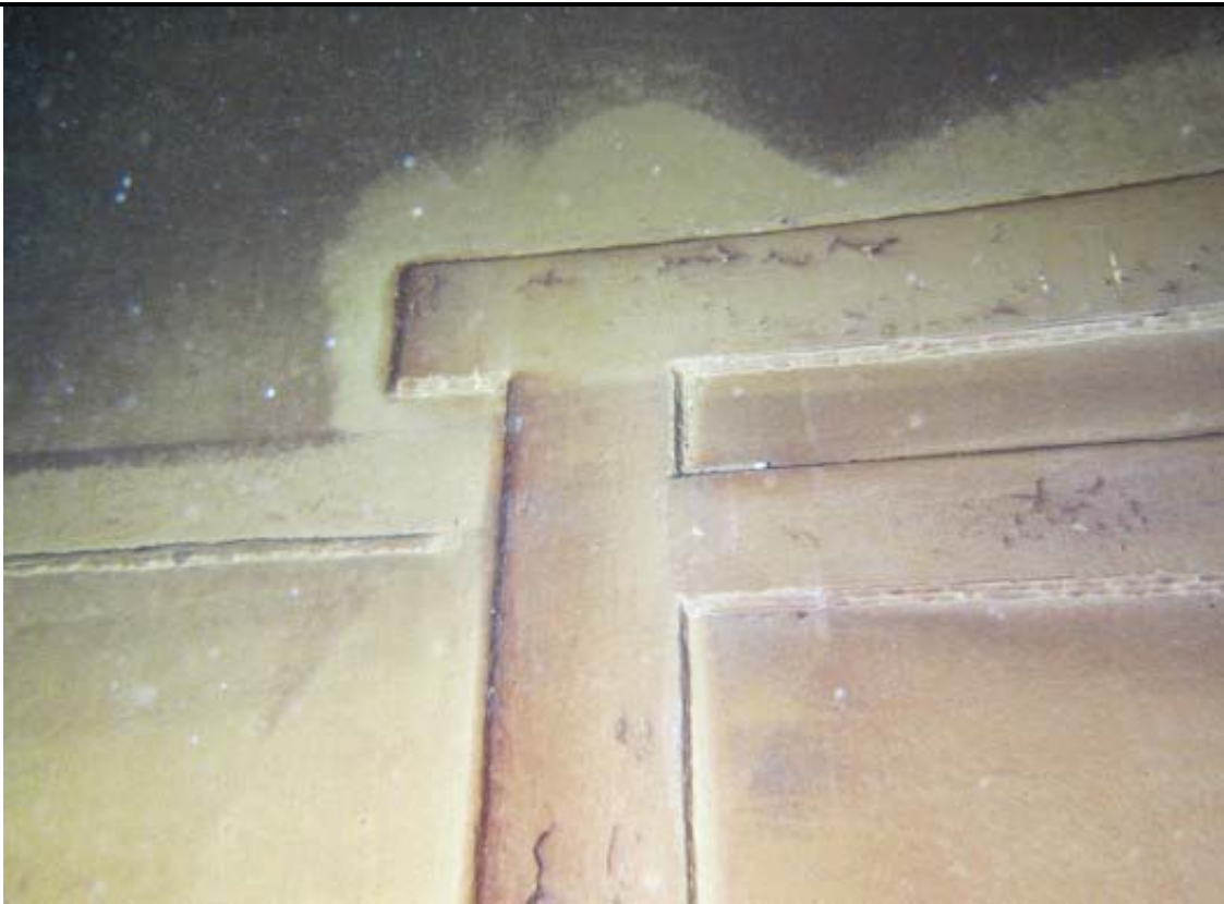
Interior shell at top corner of previous temporary shell opening ("door sheet").
