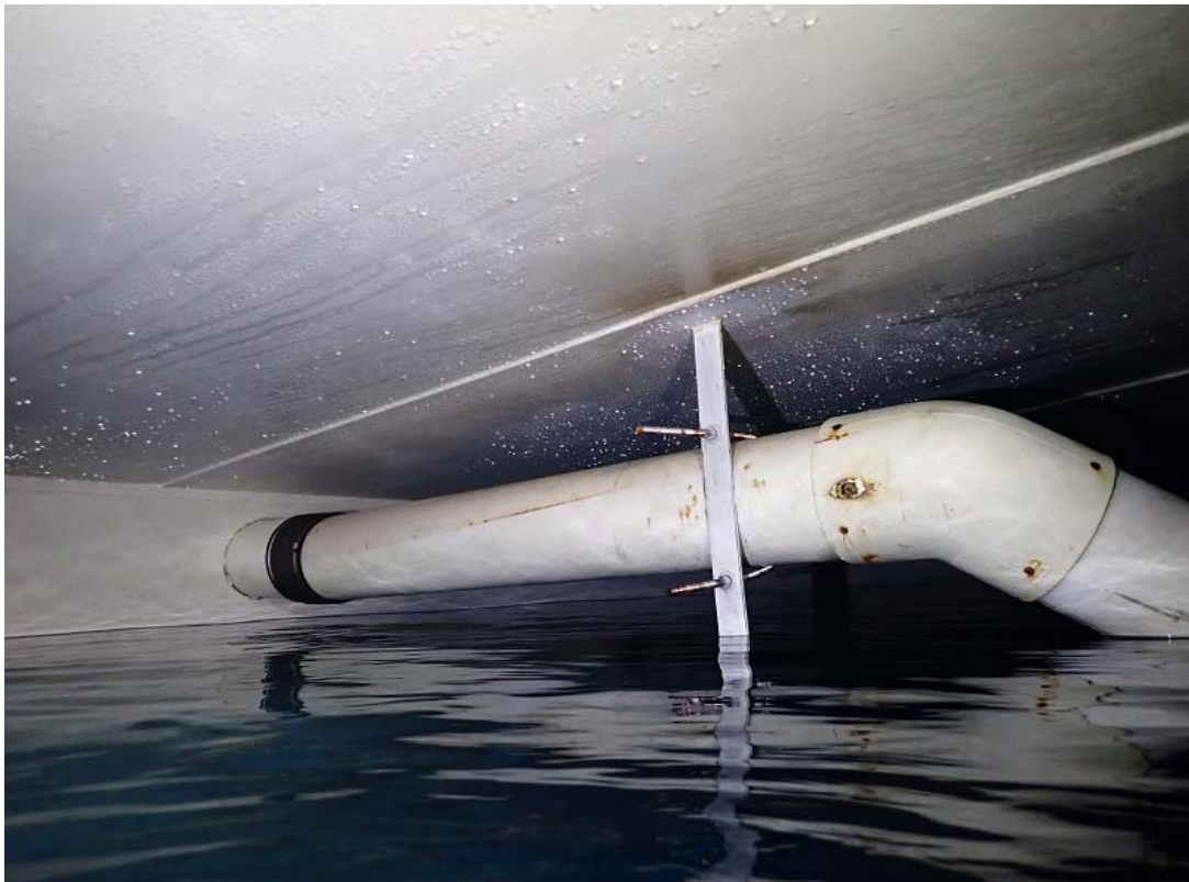
Acceptable support for PVC high inlet as shown on MG tank #1.
