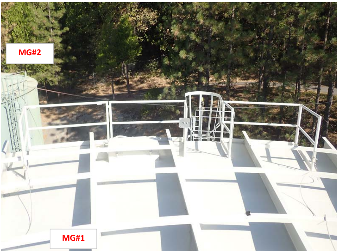
Desired roof configuration of new guardrail, and hatch at existing exterior ladder as seen on previously rehabilitated Tank #1.
