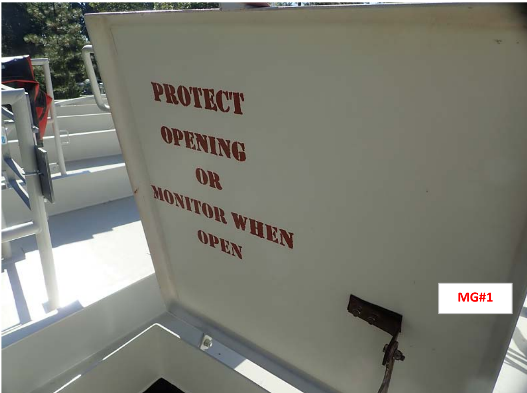
Signage required on new roof hatch.
