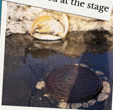
A manhole lid and liner removed by county plow
