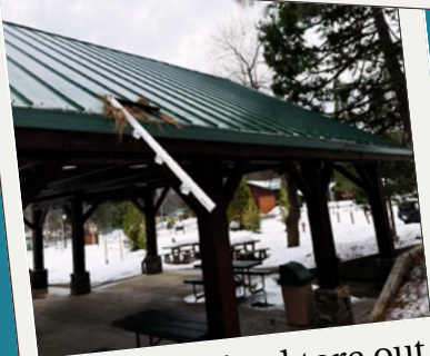
The snow load tore out the pavilion's snow cleats
