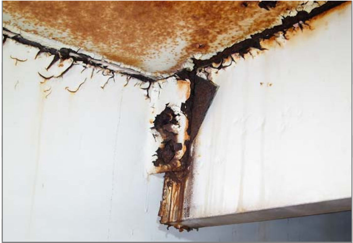
Upper shell, rafter and adjacent roof. Coatings are peeling and general corrosion is present on many surfaces.
