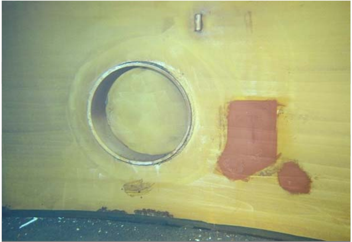
Interior view of the shell manway near quadrant 3. A spot repair is visible to the right and some significant corrosion is present below the manway.
