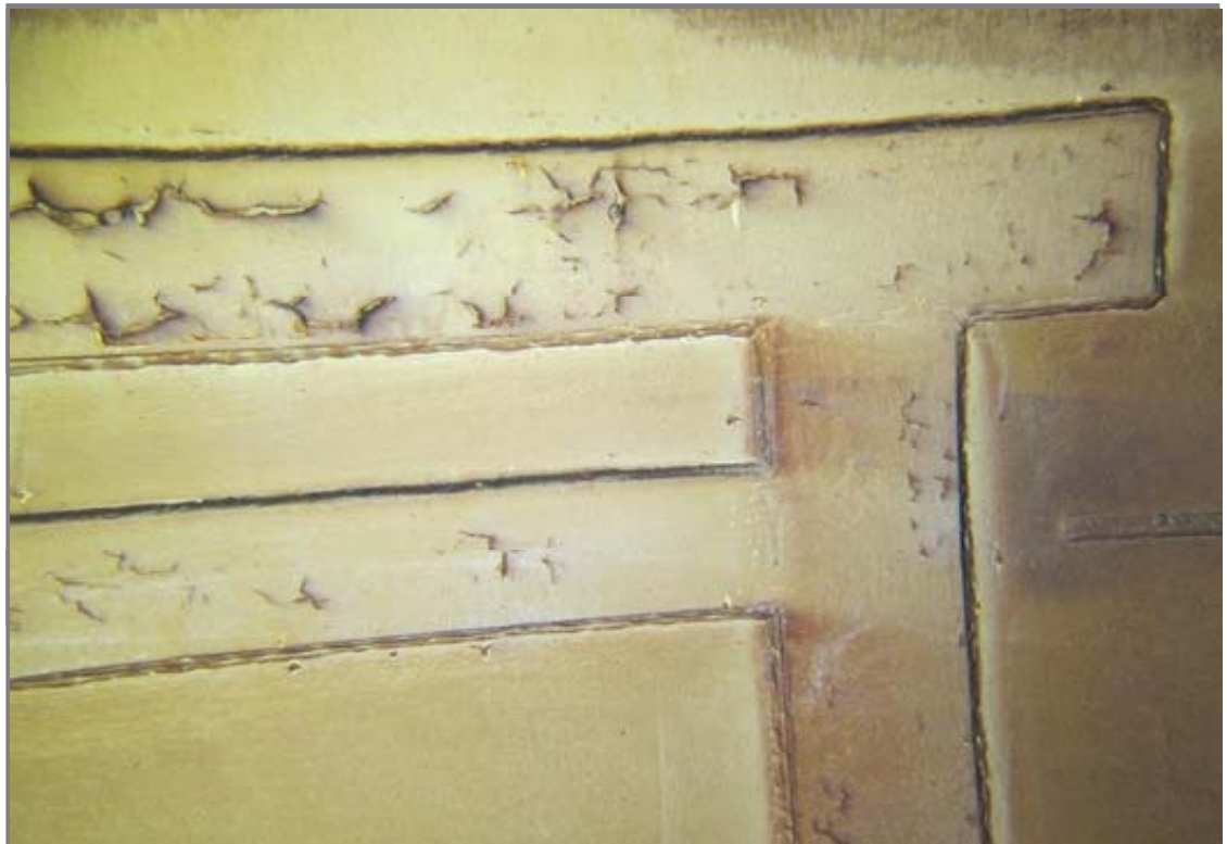
This view of cracked coatings is where a shell opening (door sheet) was cut and re-welded upon completion of the work. This area has a particularly high concentration of coating failures.
