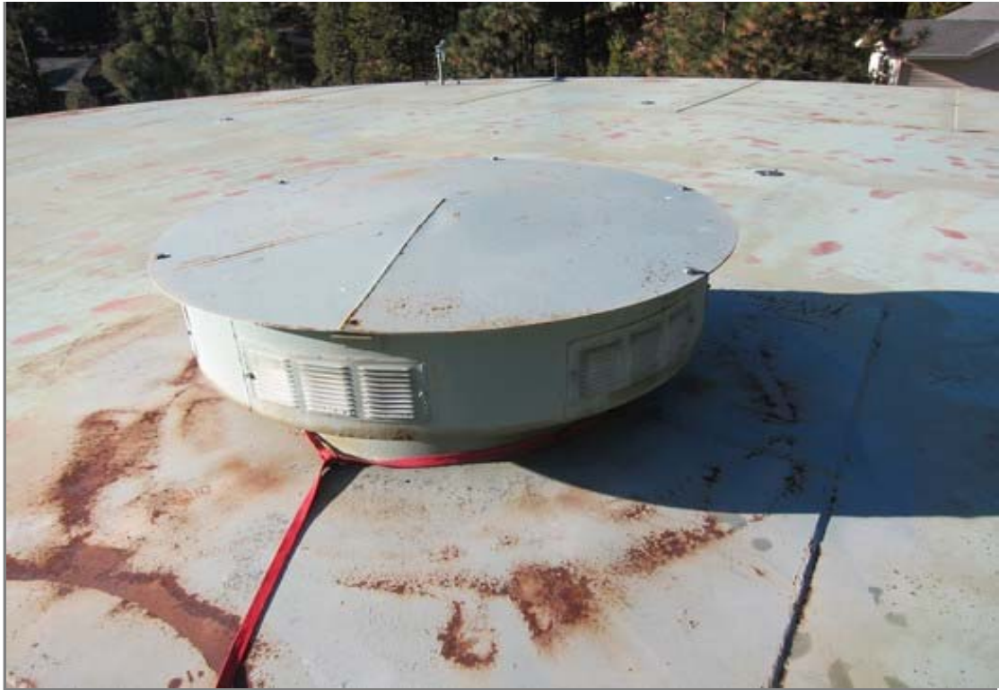
The roof vent consists of a steel cover over a steel riser pipe.
