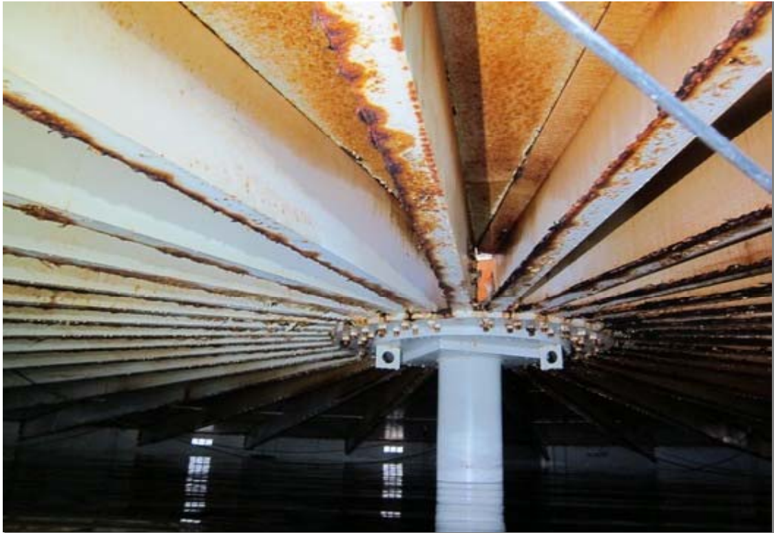
Upper center column, rafters and roof plate. Significant corrosion and associated metal loss are present.
