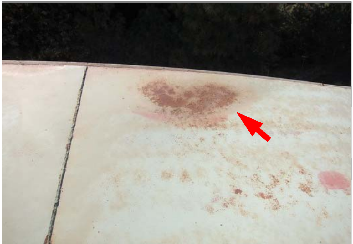
Close view of a ponding area with corrosion. Submersed exterior coatings pose a maintenance challenge.
