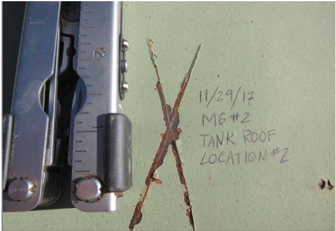
Adhesion was evaluated with a cross cut tape test and found to be 2A-3A. This location was on the exterior roof.
