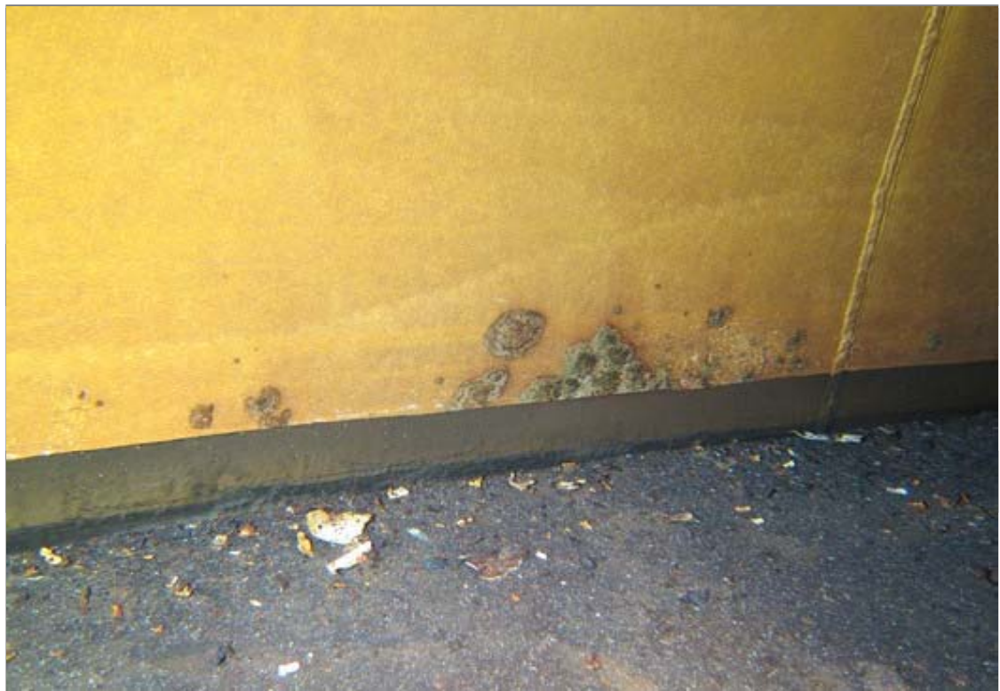
This photo shows an area of the lower shell where coatings are failing. This is an example of the worst condition in this zone.
