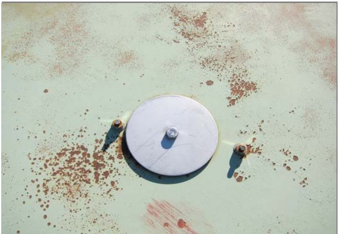
Typical view of a cathodic protection hand hole cover in good condition as viewed from the exterior roof.
