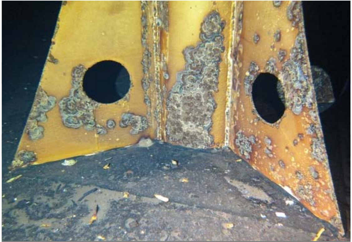
This view shows the column base plate and adjacent bottom plate. Coatings are in poor condition overall on the column and base plate.
